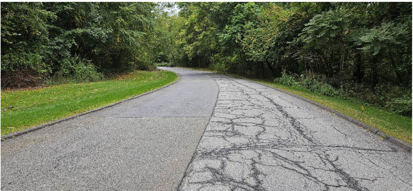
Common Roadway leading towards Armstrong Street Extensive patching and alligatored pavement.
