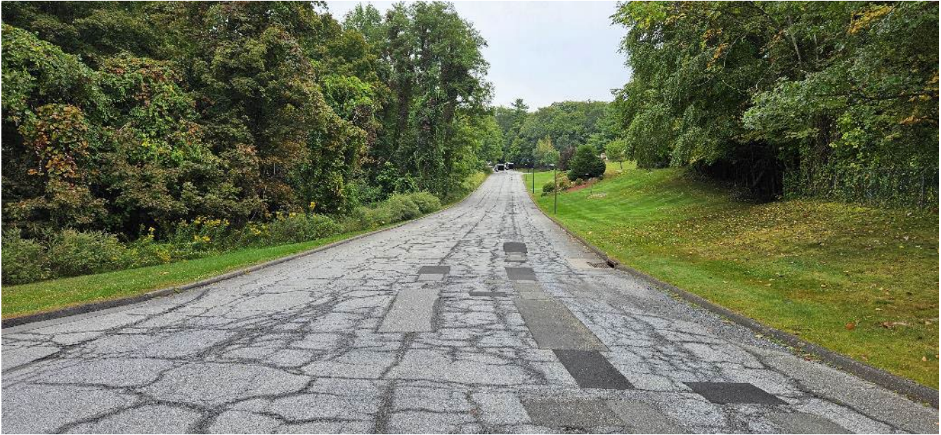
Amherst Road within development looking northeast towards Armstrong Street. Extensive patching and alligatored pavement.
