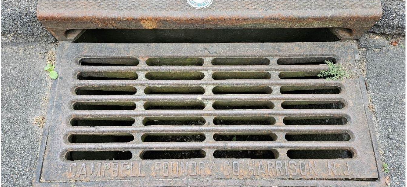
Example Catch Basin
