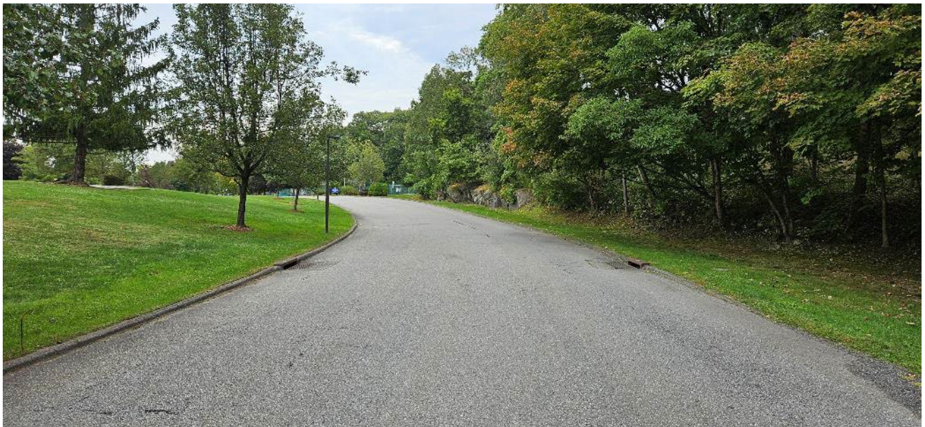
Portion of Amherst Road within development with stable but weathered pavement.
